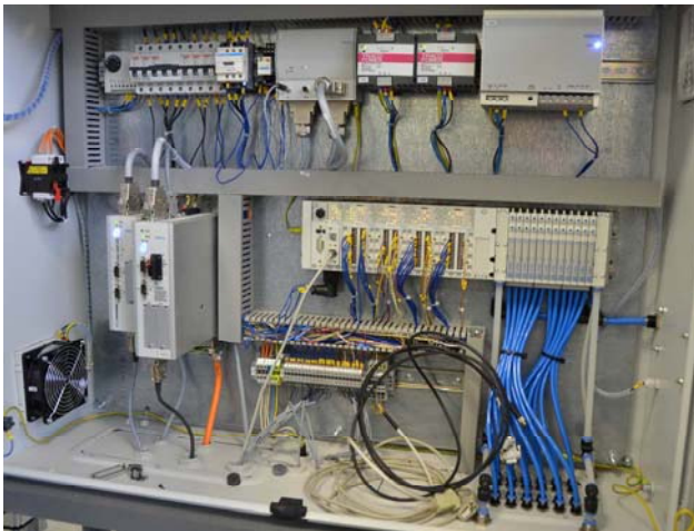
Fig. 9. Controllers and Valve Terminals for Configuration Workstation
